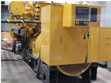
Heber Light & Power tests Cat equipment pre-market.
