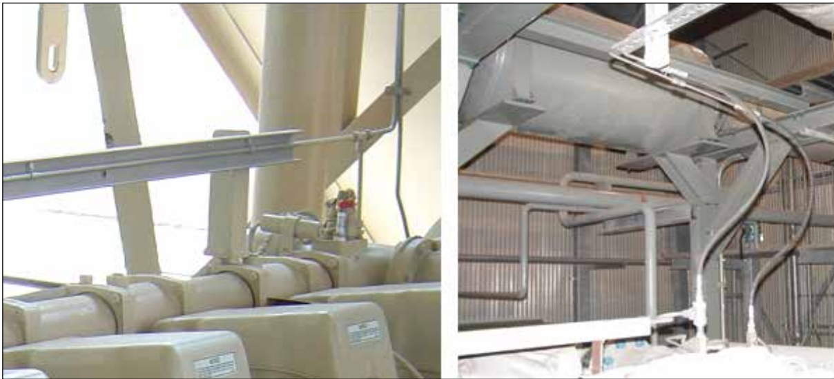
Figure 2.16 — Vent line installations showing both hard tubing and flexible hose in use.
