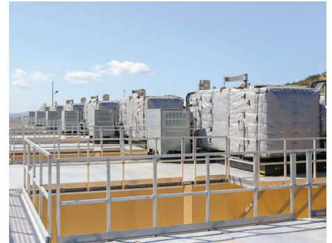
Seven Cat® CG260 generator sets consume landfill gas and create 22 MW of power to deliver to the residences, schools and businesses of Orange County.
