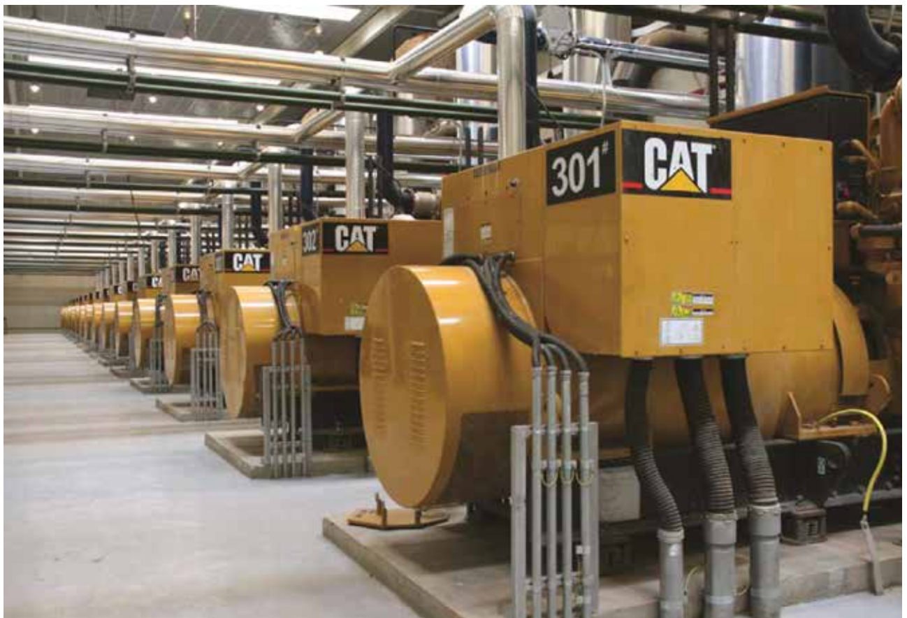
Figure 2: The interior of one of four coal gas power plants that utilize exhaust heat recovery steam generators to power a 3 MW steam turbine.
