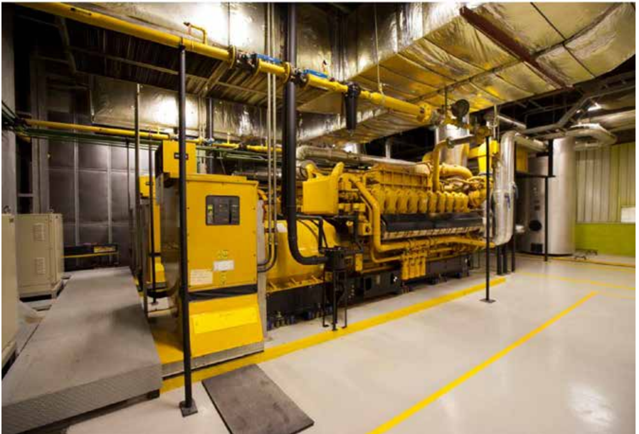
Figure 1: Four G3520C generator sets help power and cool one of the largest commercial facilities in São Paulo.
