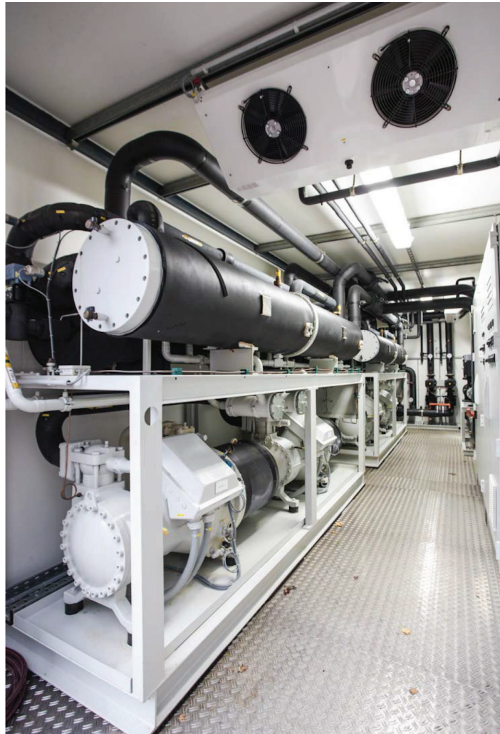
Figure 3: Industrial heat pumps installed alongside a G3516H gas generator set in a district energy plant in Reutlingen, Germany
