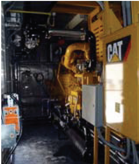
Since installation in August 2011, the Cat® G3516 has run 3,000 hours at an average of 98 to 99 percent capacity, with downtime only for utility outages or routine maintenance.
