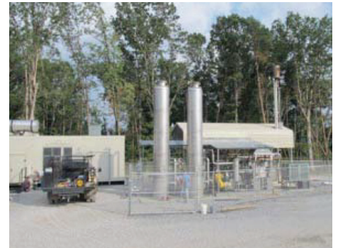
The completed landfill gas-to-energy plant at the Alcoa Landfill is converting 95 percent of recovered methane gas to power, generating enough electricity to power approximately 750 homes.
