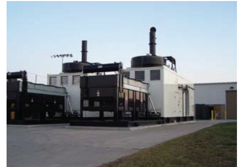
The G3520E and G3516H generator sets are housed in outdoor enclosures. The building in the background houses entire electrical and mechanical infrastructure required to operate in parallel with LEC's electric utility feed.
