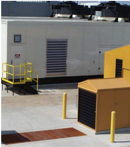
The energy produced during product testing at the Endurance Facility – located on the Lafayette Engine Center (LEC) in Lafayette, Indiana – is helping to power LEC and contributing toward Caterpillar’s corporate sustainability goals.
