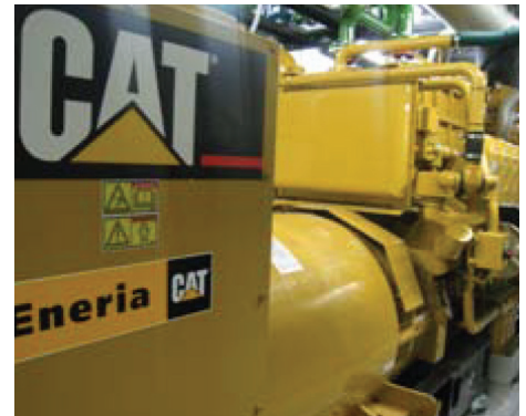
This Cat® G3508 gas generator set has been supplying 50 percent of the treatment plant's power needs since 2005.
