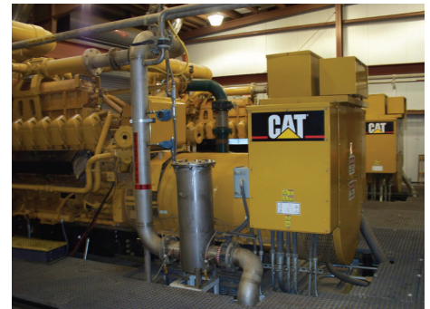
Cat® G3520C Landfill Gas Low-Emission generator sets at the Seminole Road Landfill
