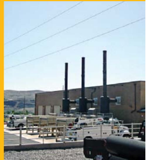
Hurricane City Power Plant
