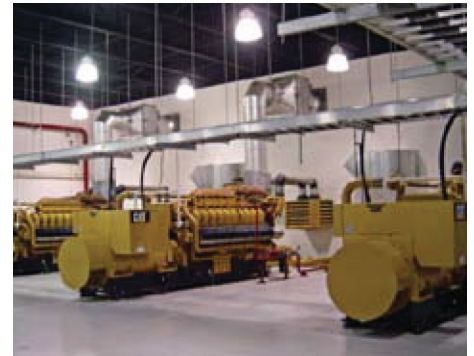
Three Cat® G3520C high voltage gensets @ 2050 ekW each.
