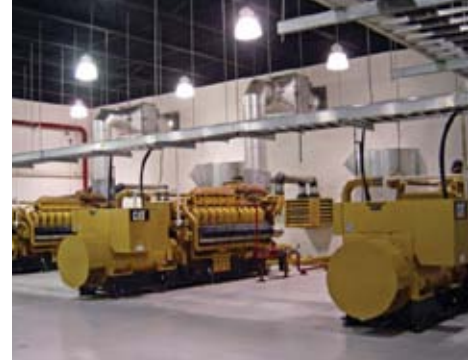
Three Caterpillar G3520C High Voltage Gensets @ 2050 kW each.
