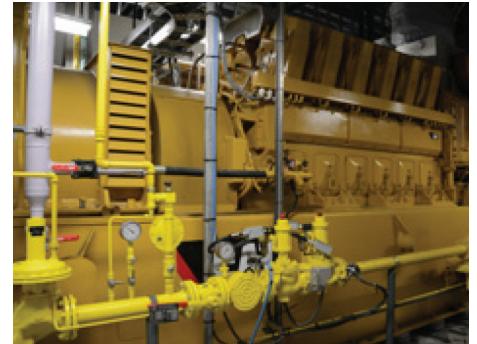
Cat® CG260-12 natural gas generator set installed at Markham District Energy's Birchmount Energy Centre for its combined heat and power (CHP) application.
