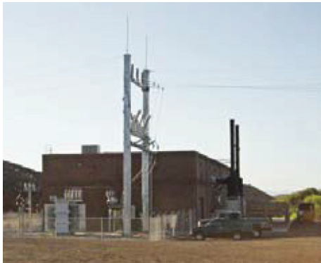
Fort Clara Power Plant
