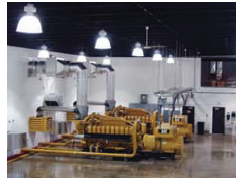
Phase 1 of power plant construction. Two Cat® G3520C high voltage gensets @ 2050 kW each.
