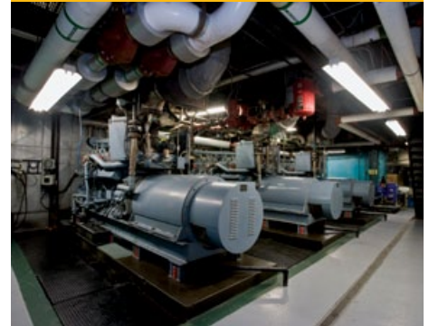
The three generator sets powered by Cat® G399 engines at Snowbird have each passed 200,000 hours of service.
