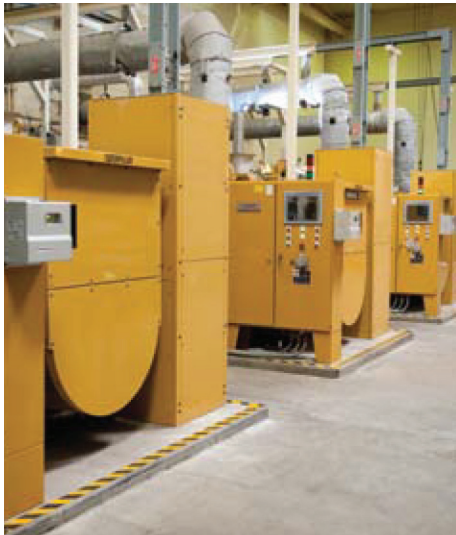
The biogas produced by the water treatment process at the Encina Water Pollution Control Facility fuels four Cat® G3516 engine generator sets for renewable energy.
