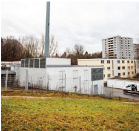
Since installing the new Cat® G3516H engine, HBG has experienced significant efficiency improvements. The G3516H, in combination with the heat pump, increased plant efficiency to 103.7 percent.
