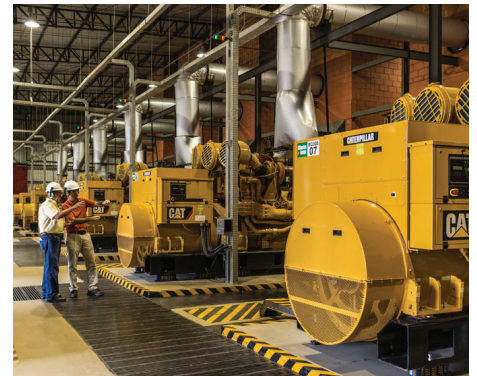
The Monte Cristo power plant uses 34 Cat® C175-20 diesel generator sets to supply 3150 kW of gross power to the Boa Vista area.
