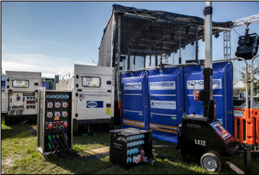
Two 200 kVA generator sets providing prime and standby power to a festival stage in Somerset, UK.
