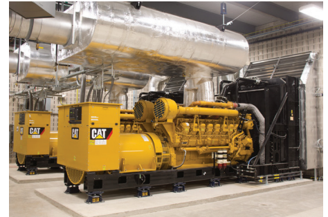
Patten Cat installed two Cat® 3516 diesel generator sets with a dual-silencer system and paralleling switchgear to meet power generation and sound requirements at Edward Hospital.
