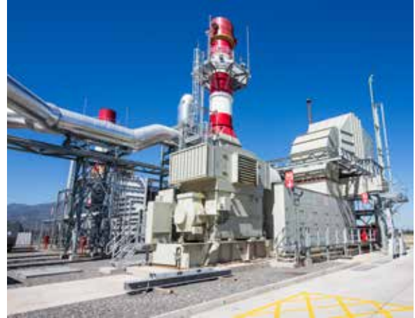
Titan 250 Generator Set - Chile
