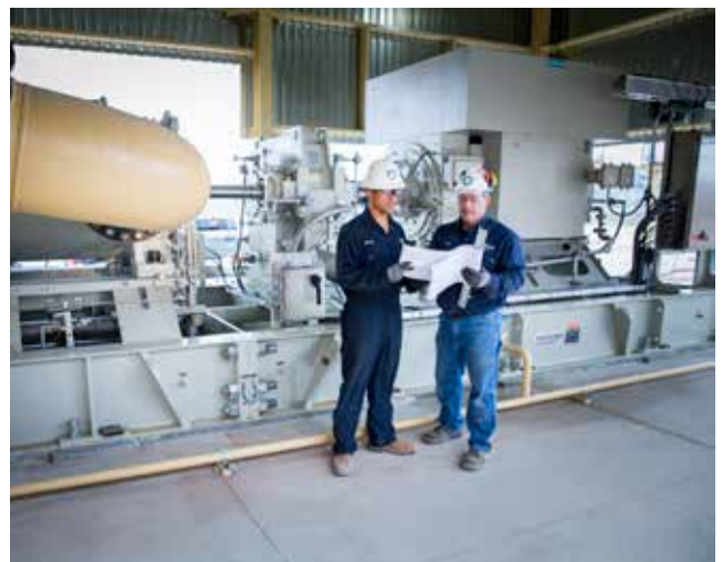
Electric Motor Drive, C33 Compressor - USA
