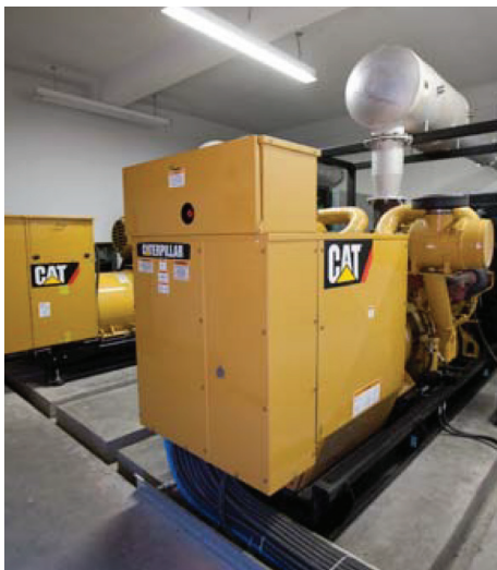
Cat® diesel generator sets supply standby power for Condaspar's factory operations and also allow the company to engage in peak shaving activities during evening hours when power is most expensive.
