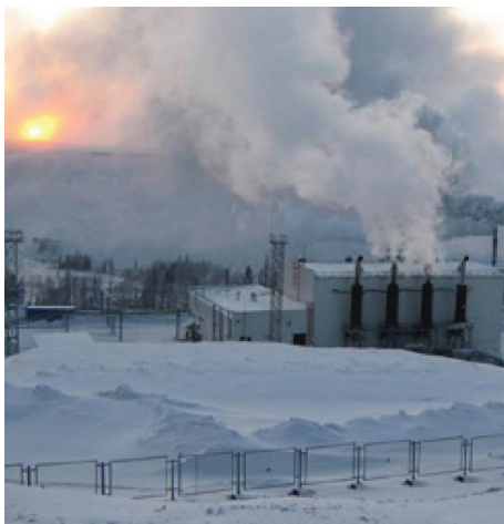
With winter temperatures reaching -50°C, building oil pipelines is not a practical way to supply energy to remote regions of Russia. Instead, crude oil delivered by truck from local oil fields is used to fuel Cat® generator sets.
