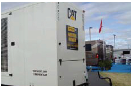
Whayne Power Systems installed three Cat® 3516B diesel generator sets for 6.75 MW of power to provide up to two weeks of emergency backup power in the case of a power outage.
