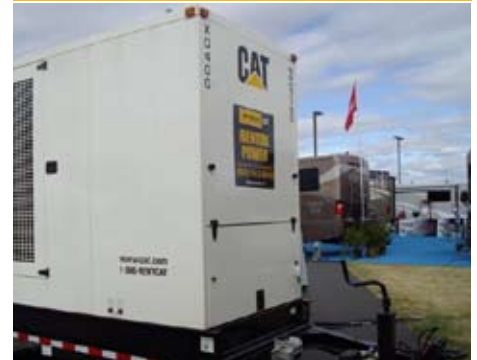
Hale Northeastern Exposition Services provides on-site temporary power for national recreational vehicle rally.
