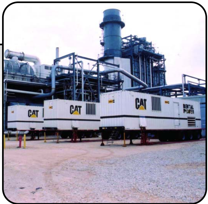
Three Cat XQ2000 Power Modules provided up to 6 MW of temporary power to the Guadalupe Power Plant during scheduled substation maintenance.
