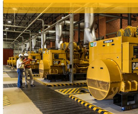
The Monte Cristo power plant uses 34 Cat® C175-20 diesel generator sets to supply 3150 kW of gross power to the Boa Vista area.
