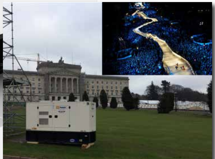
Rental generator set supporting Red Bull Crashed Ice event at Stormount Estate, Belfast , Northern Ireland.
