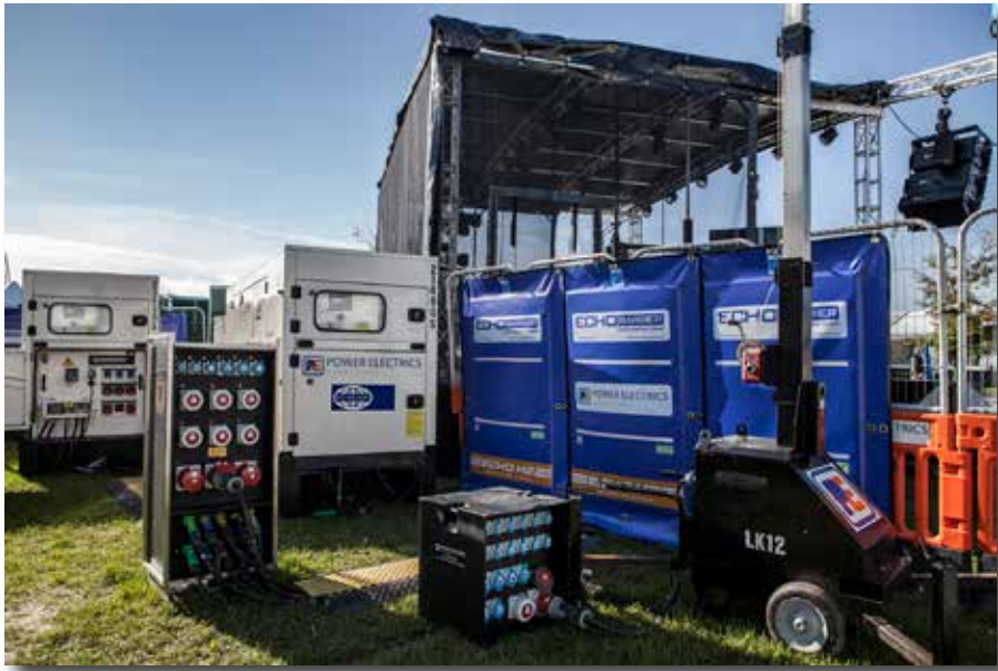
Two 200 kVA generator sets providing prime and standby power to a festival stage in Somerset, UK.
