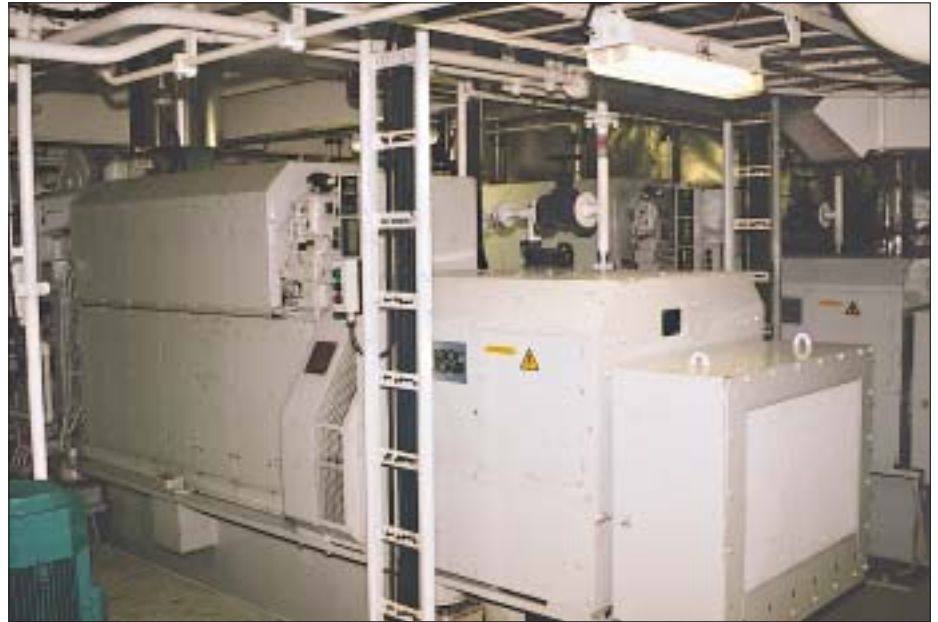
Electric power is derived from three MAN Holeby 6L 16/24 gensets, each developing 515 kW
