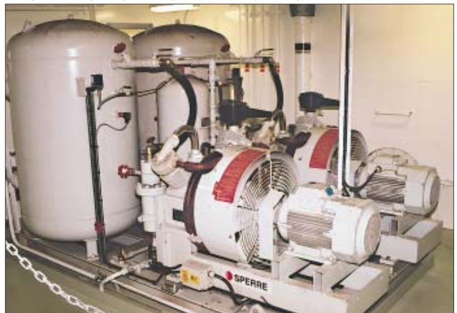
Starting air for the engines is generated by two Sperre air compressors, type HL2/120
