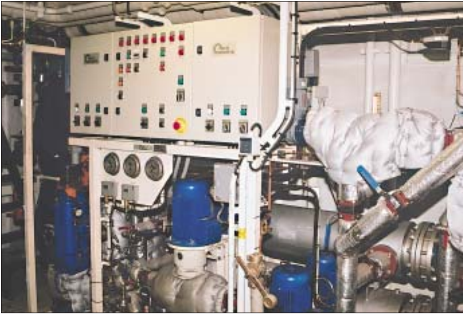
Fuel oil conditioning is carried out with a Mar-In Controls fuel oil supply module
