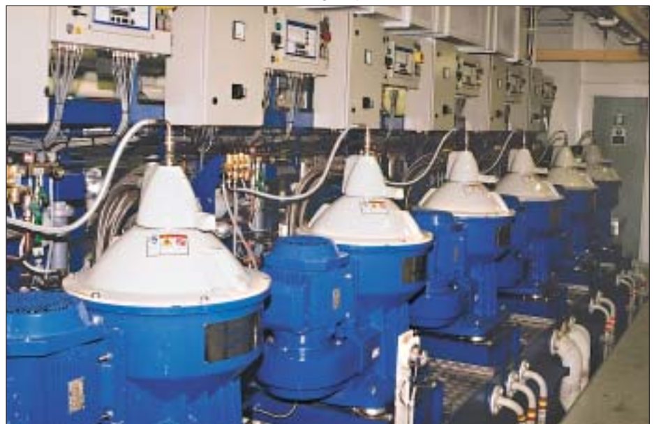
Fuel oil and lube oil treatment is with Alfa Laval centrifugal separators
