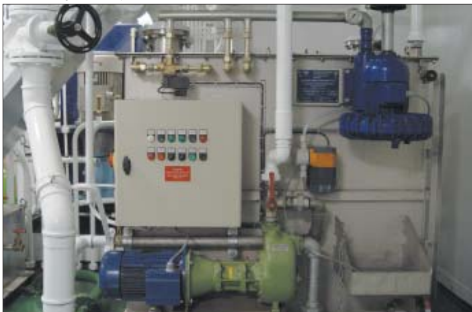
The DVZ sewage treatment plant
