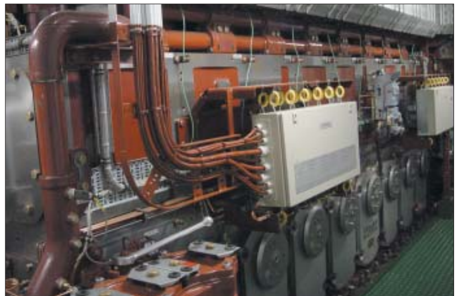
The propulsion plant consists of a MaK 8M32 medium-speed main diesel engine
