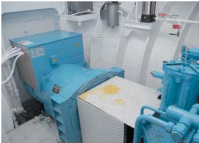
A Stamford shaft generator is used when sailing
