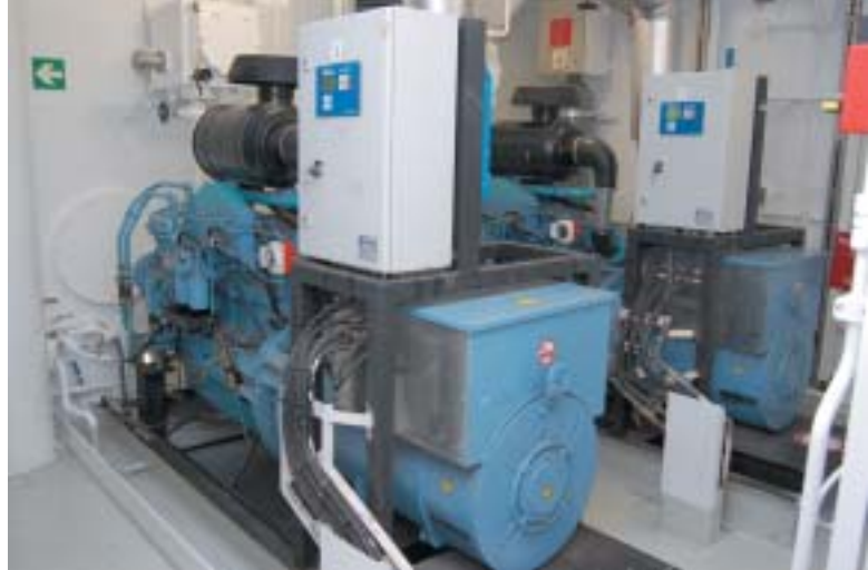
Sandfirden delivered the gensets
