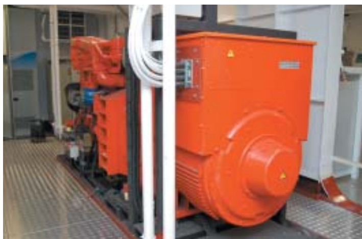
Caldic supplied the alternators for the gensets
