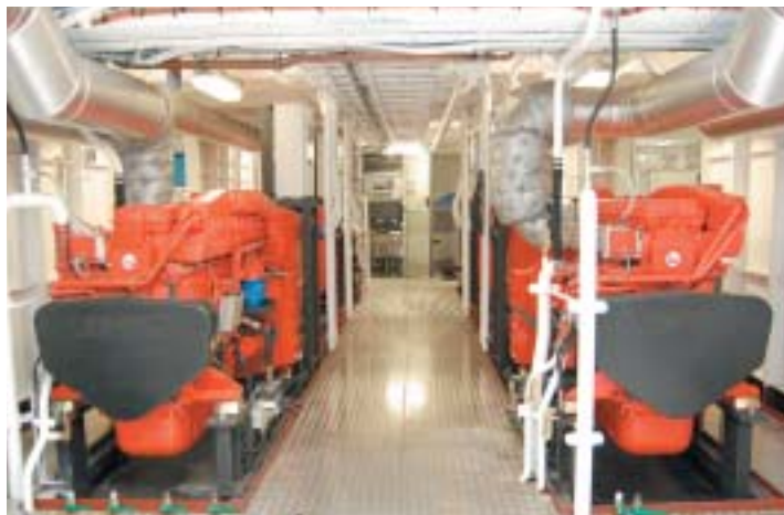
Four gensets are located in the spacious engine room
