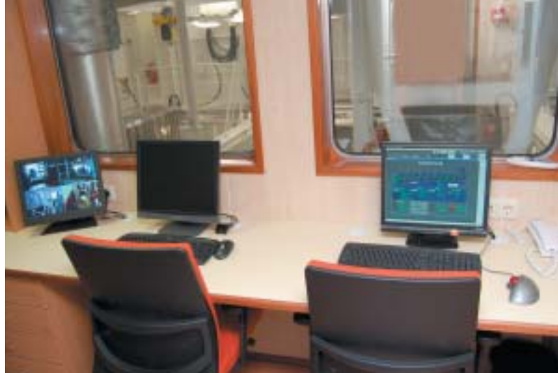
The alarm and monitoring system is accessible through TFT screens
