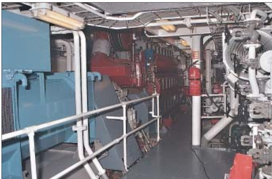
The vessel's propulsion plant features two MaK 9M25 four-stroke marine diesel engines
