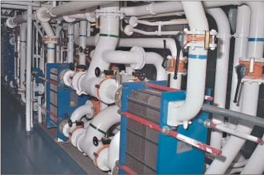
The cooling water system features Alfa Laval plate heat exchangers
