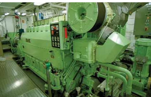
A single MaK 8M20 main engine drives a Scana Volda CP propeller
