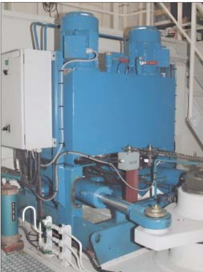
Directional control is with a Promac hydraulically powered steering gear
