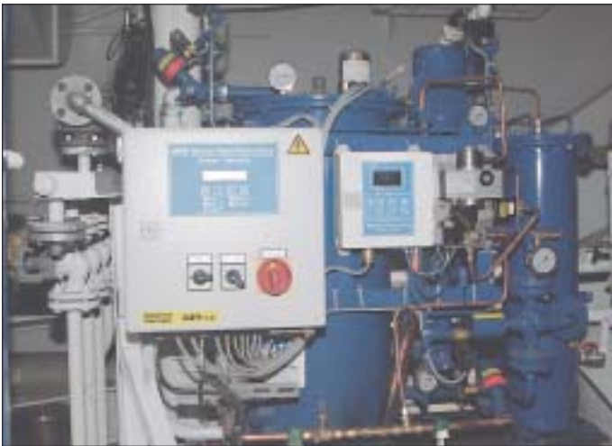
The RWO oily water separator
