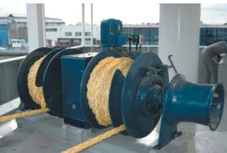
On the aft ship two electric hydraulic mooring winches are installed
