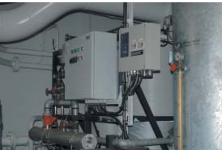
The Hatzenboer-Water fresh water treatment
