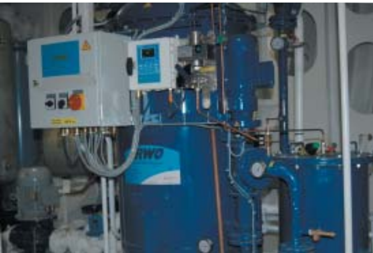
The RWO bilgewater separator
