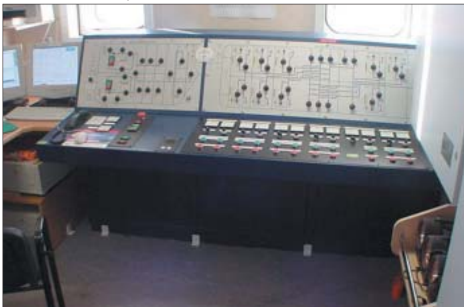
The control console in the cargo control room
