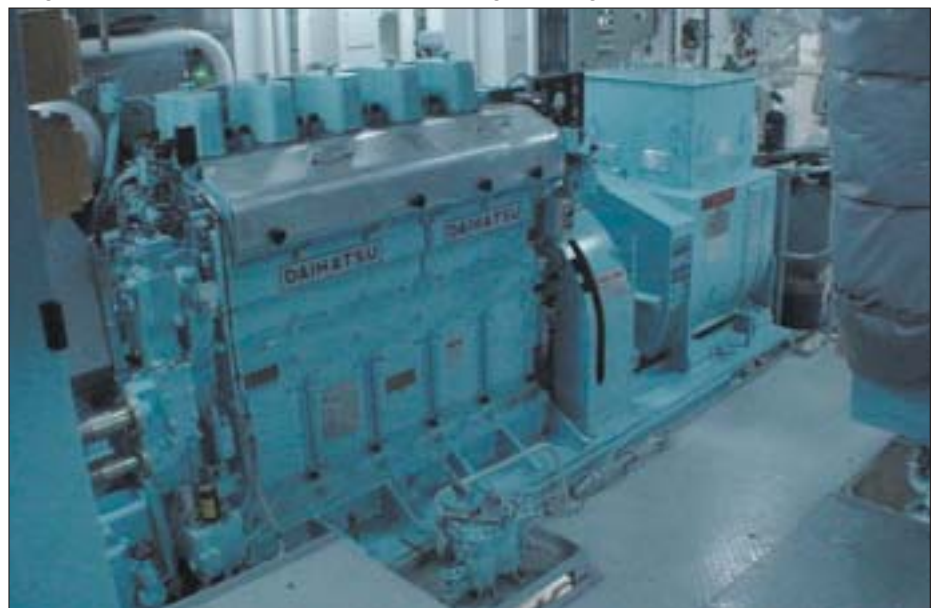
The generator sets consist of 420 kW Daihatsu diesel engines driving a brushless alternator
