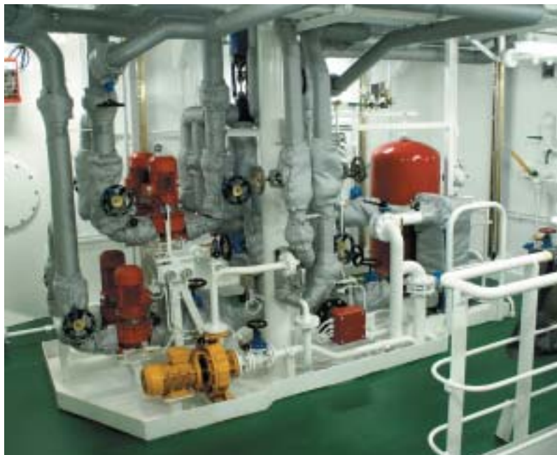
*The hot water generating plant
