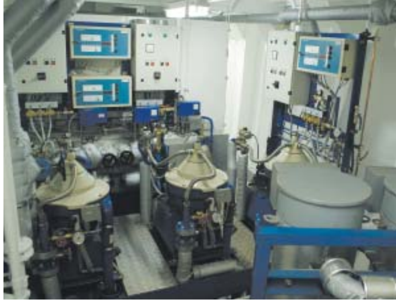
Fuel is treated in a dedicated separator room
