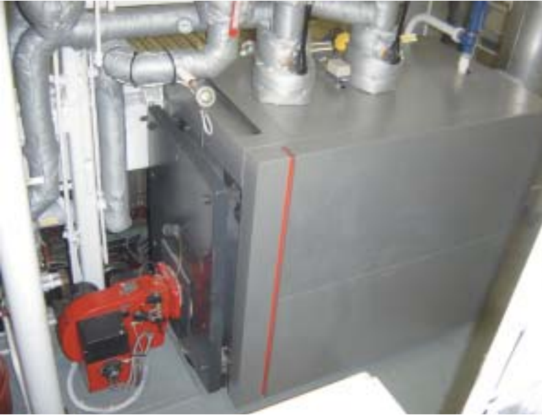
The Heatmaster boiler
