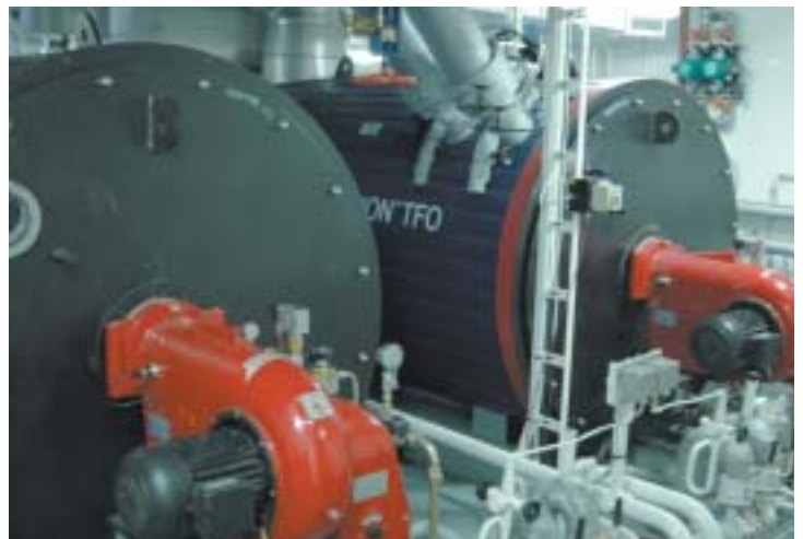
The Aalborg Industries thermal fluid heating units
