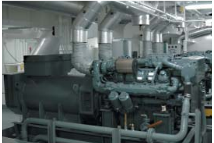
Auxiliary power is derived from three MAN diesel-driven alternators
