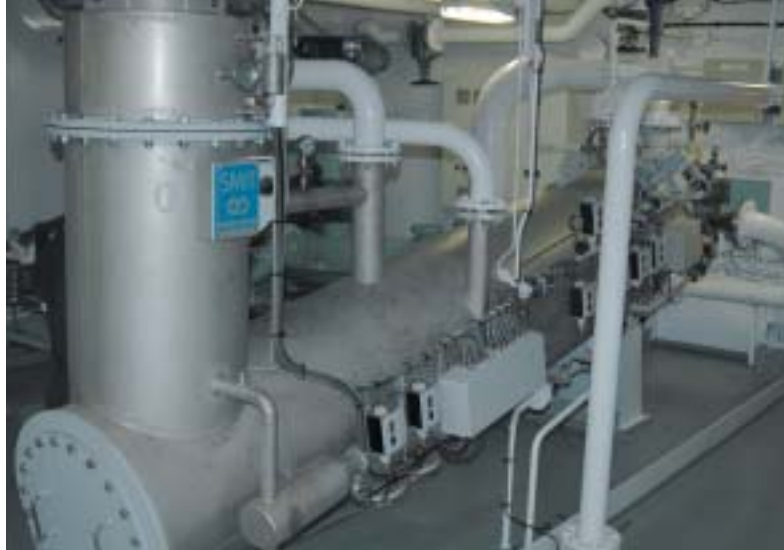
Gas freeing of the tanks is executed with a Smitgas Systems inert gas generator
