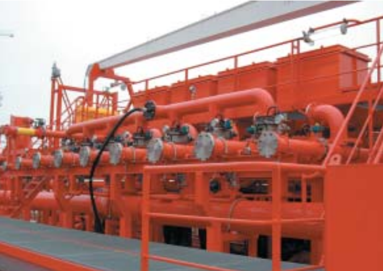
Eight cargo segregations have been provided with individual cross-overs
