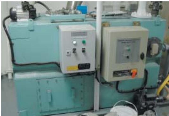
The Hamworthy KSE sewage treatment plant
