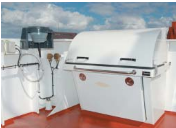
The bridge wings are equipped with navigation consoles
