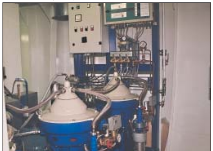
The Alfa Laval oil separator plant
