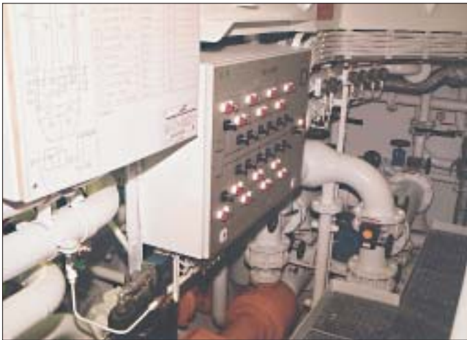
The ballast system is remote controlled from a control cabinet in the engine room
