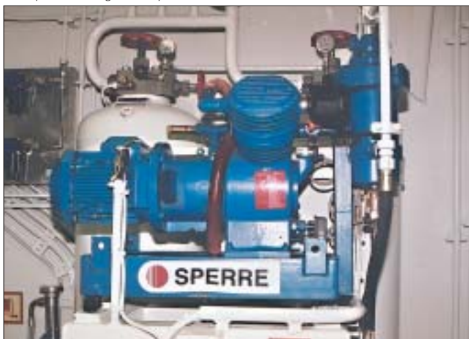
The Sperre starting air compressors
