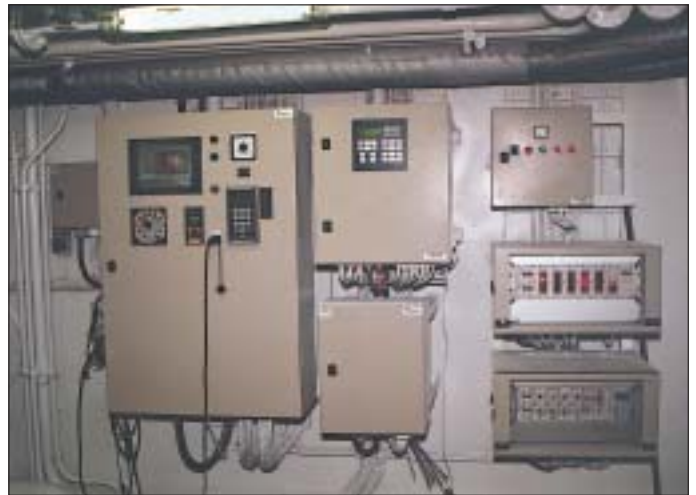
Teh alarm- & monitoring system was supplied by Alewijnse Noord
