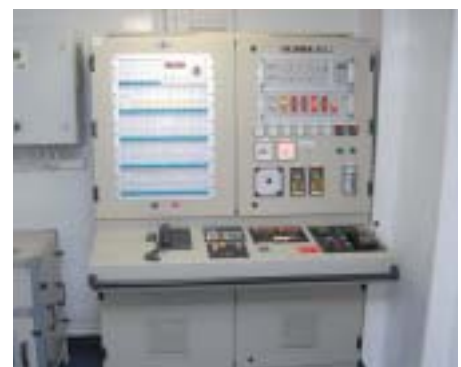
The electrical installation was done by Alewijnse
