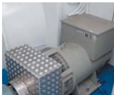
The shaft generator is from Leroy Somer
