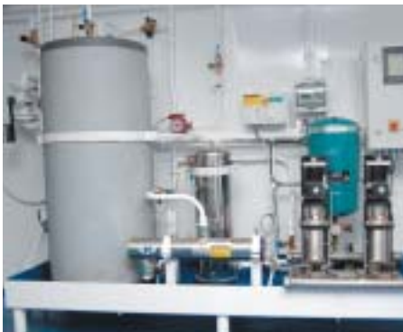
Water treatment is with Hatenoer equipment
