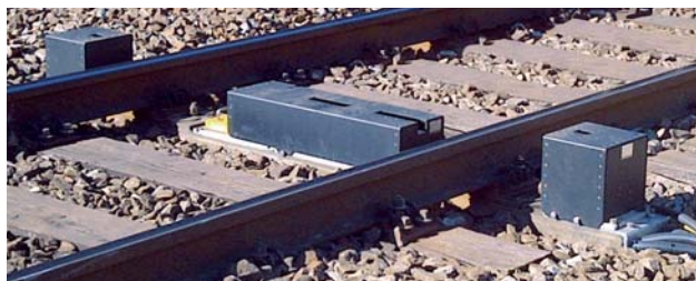
FUES-EPOS installation with snow covers in Switzerland
