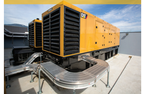
Two Cat C32 diesel generator sets provide backup power for the data center building and the infrastructure to support 50 high-density server racks.
