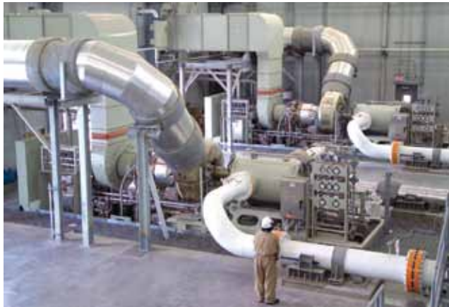
C40 Gas Compressor
