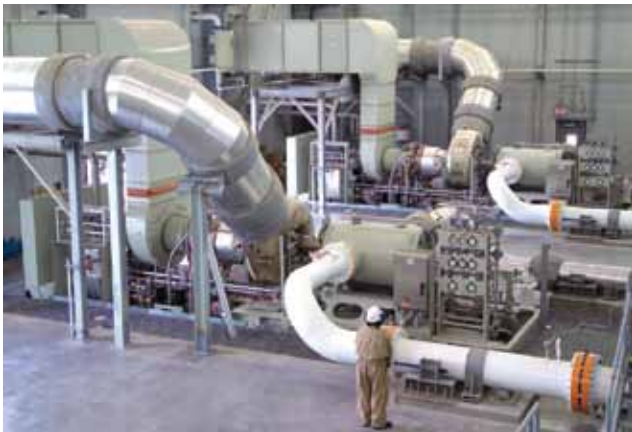
C40 Gas Compressor
