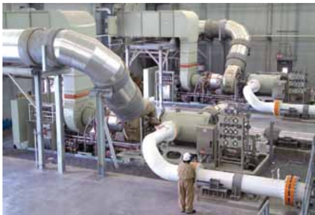
C40 Gas Compressor
