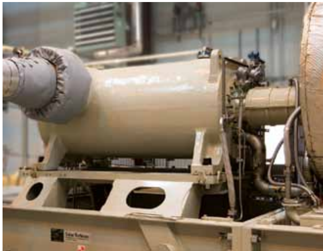
C61 Gas Compressor
