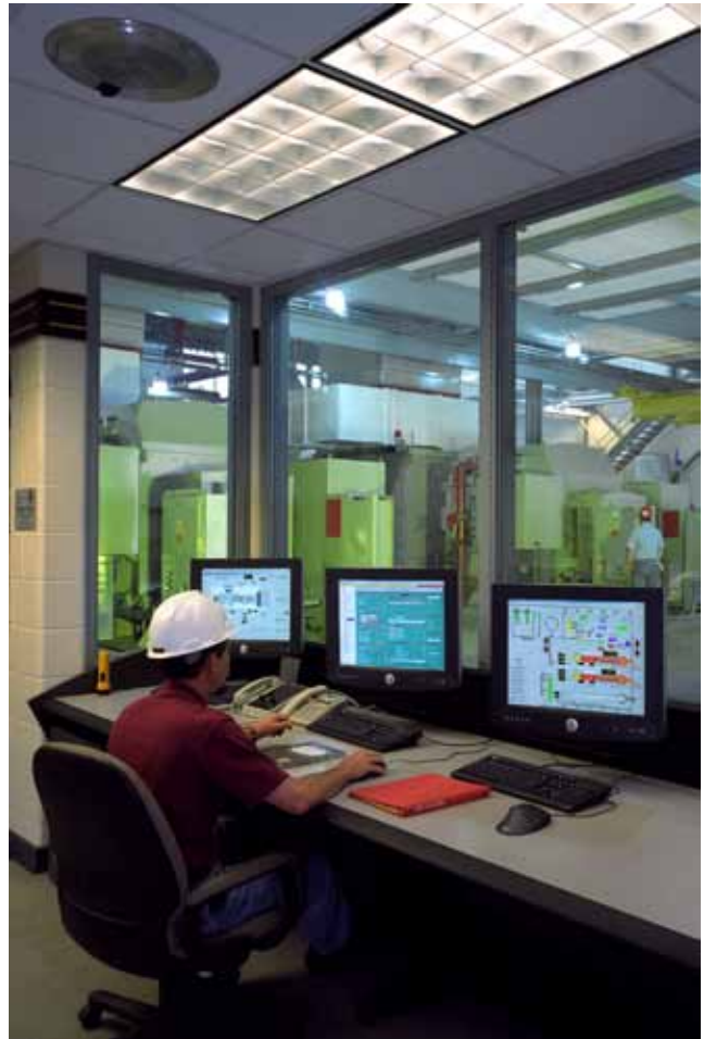
Titan 130 Generator Sets - Missouri, USA
