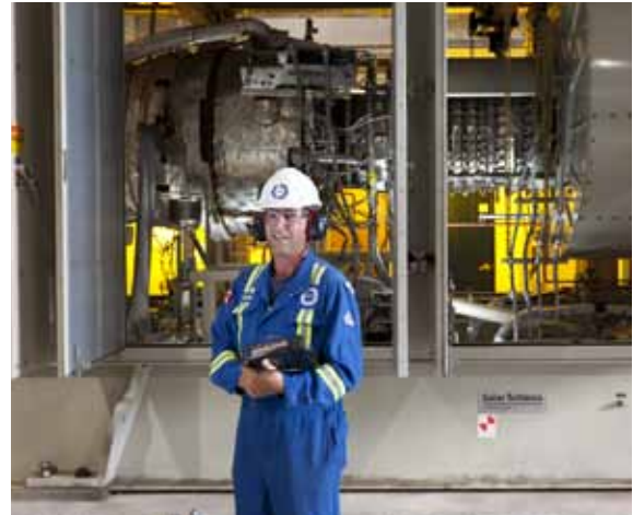
Titan 130 Generator Set - Ontario, Canada
