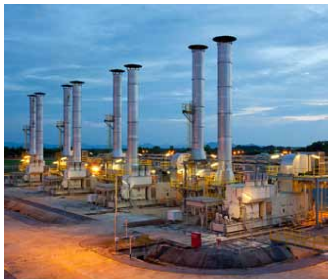
Mars 100 Mechanical-Drive Packages - Songkhla, Thailand
