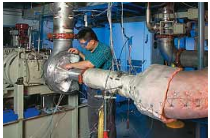
San Diego Compressor Aero Test Facility
