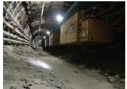
Cat VFD system underground
