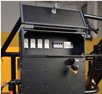
High-powered generator easily powers nighttime lighting configurations.
