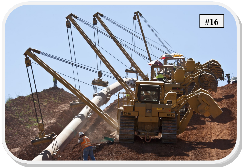
This team of PL87 Pipelayers work together to haul a long piece of pipe uphill.
